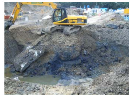
Figure 4 - Contamination around Culvert
